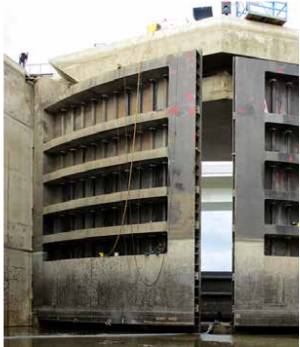
Gate of the Lanaye lock
