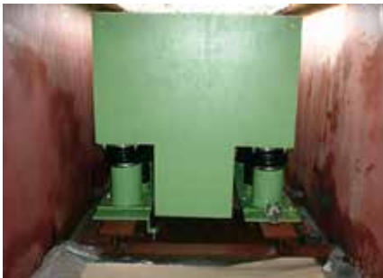
Tuned mass damper (TMD)
